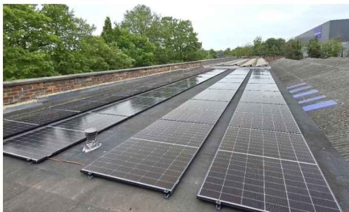
Figure 12. SPS Training Solutions' Solar PV installation funded by the Green Business Grant.
