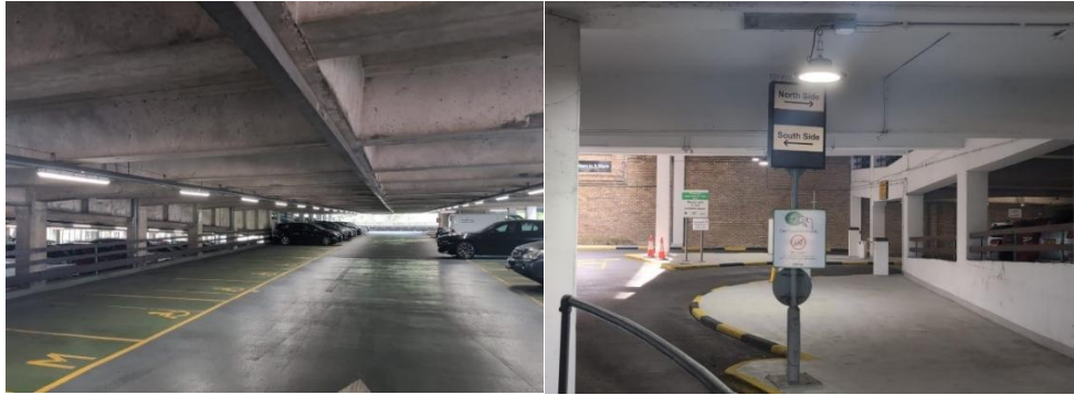
Figure 27. St George's MSCP new efficient LED lighting system.
